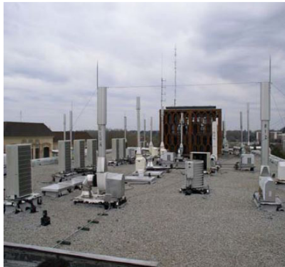
Roof-mounted exhaust fans, stacks, and condensing units
