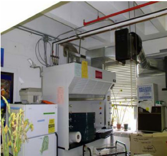
Typical auxiliary air lab fume hood with non-conditioned air ventilation
