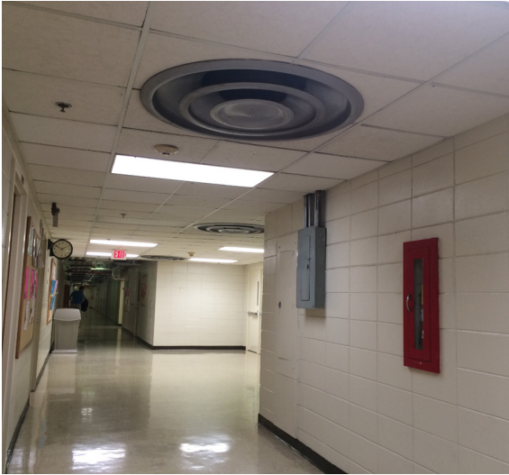
Large diffuser in hallway supplies ventilation to central building
