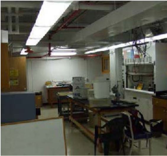
Lab fan coil units limit overhead space
