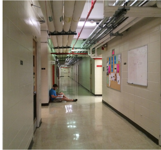
Mechanical systems exposed in hallways
