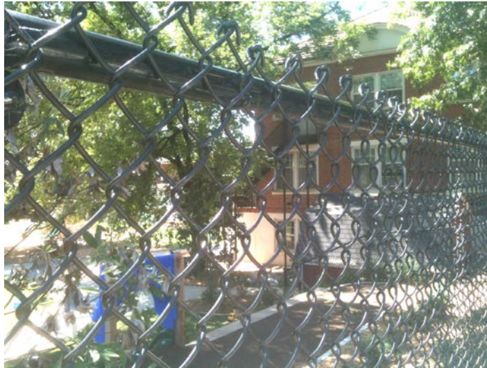
Chain-Link Fence – McPhaul Child & Family Development Center
