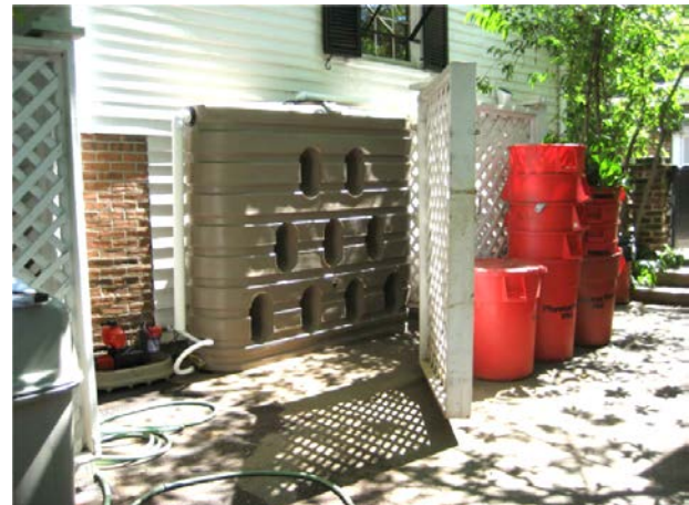
Above-Ground Cistern – Founders House
