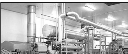
Potato Chip Manufacturing Facility
