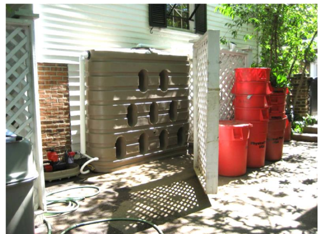
Above-Ground Cistern – Founders House
