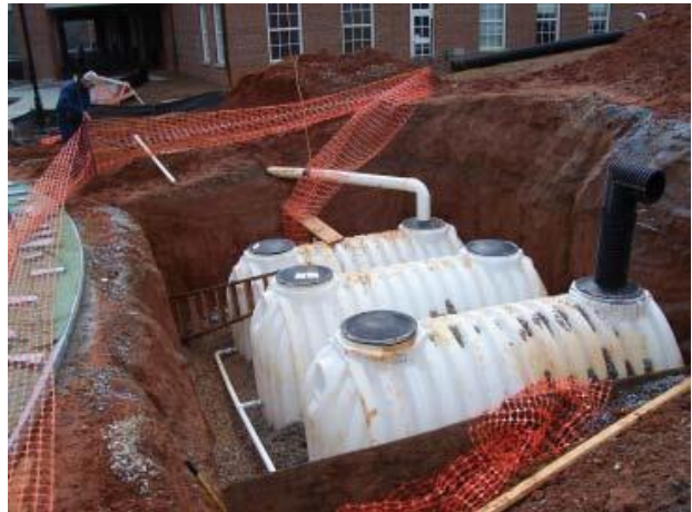
Underground Cistern – Miller Learning Center
