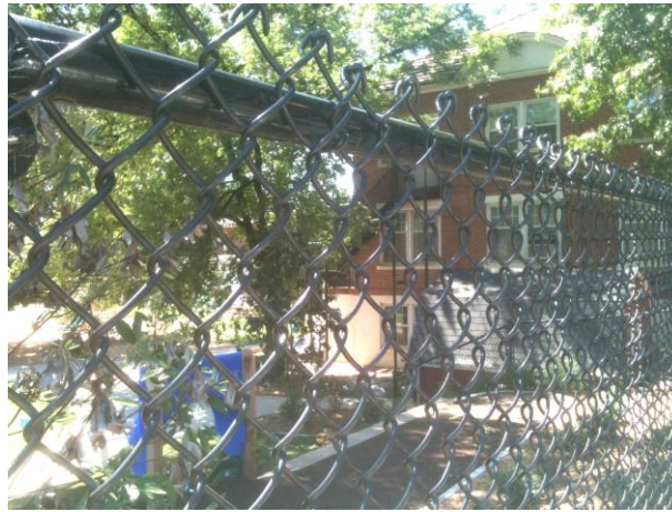
Chain-Link Fence – McPhaul Child & Family Development Center
