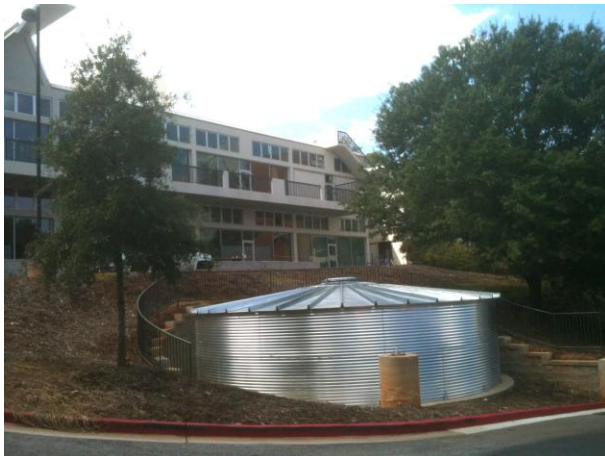
Above-Ground Cistern – Jackson Street Building
